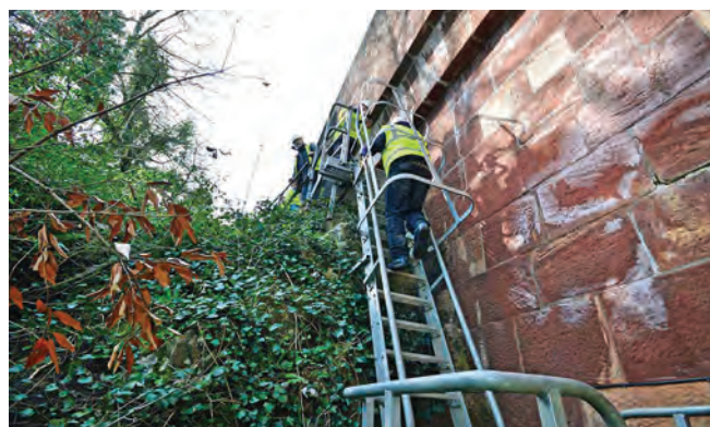
Access ladder down to entrance chamber entrance recently cut by the Bridge Trust through the 2m thick red sandstone abutment wall
